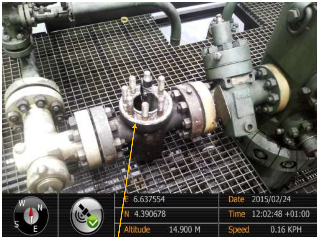
Close-up: Position of missing Control Unit on Belema Well10L Wellhead at Belema. Picture was taken during Joint Investigation of 24 th February 2015.
