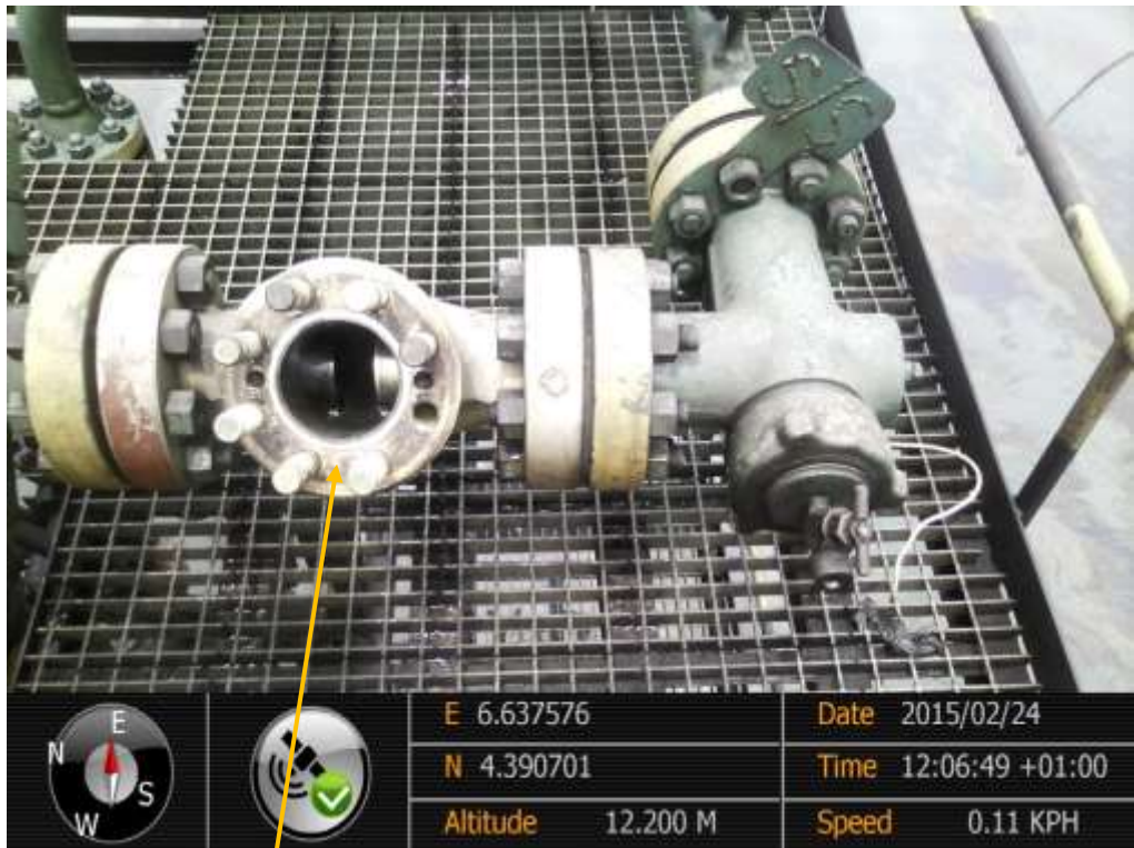
Close-up: Position of missing Control Unit on Belema Well10S Wellhead at Belema. Picture was taken during Joint Investigation of 24 th February 2015.
