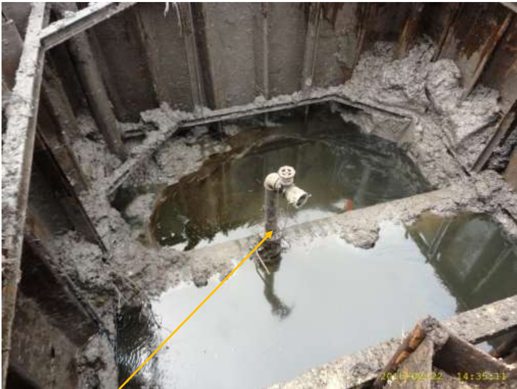
Close-up: Illegal fitting on 28" Bomu-Bonny Pipeline at Bodo West. Picture was taken during Joint Investigation of 22 nd February 2015.
