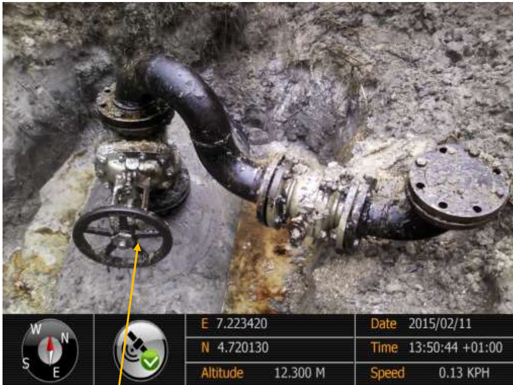
Close-up: Illegal fitting on 28" Nkpoku-Bomu Pipeline at Kpoghor/Gbam. Picture was taken during Joint Investigation of 11 th February 2015.
