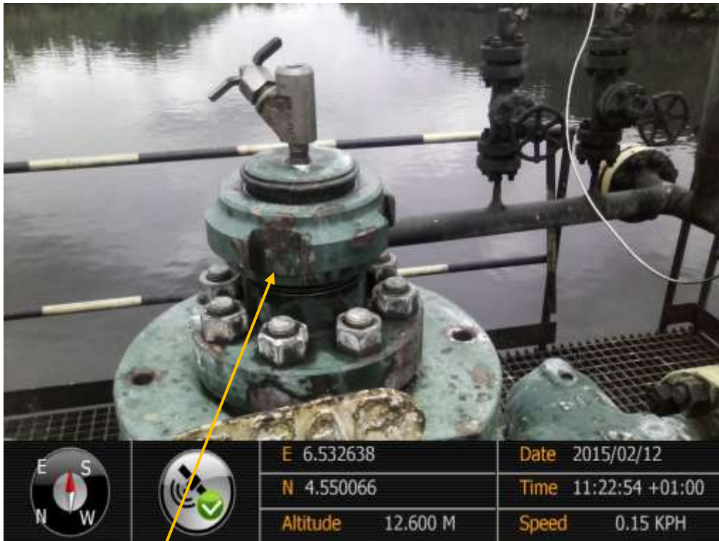
Close-up: Tampered tree cap cover on Santa Barbara Well21T Wellhead at Nembe/Bassambiri. Picture was taken during Joint Investigation of 12 th February 2015.
