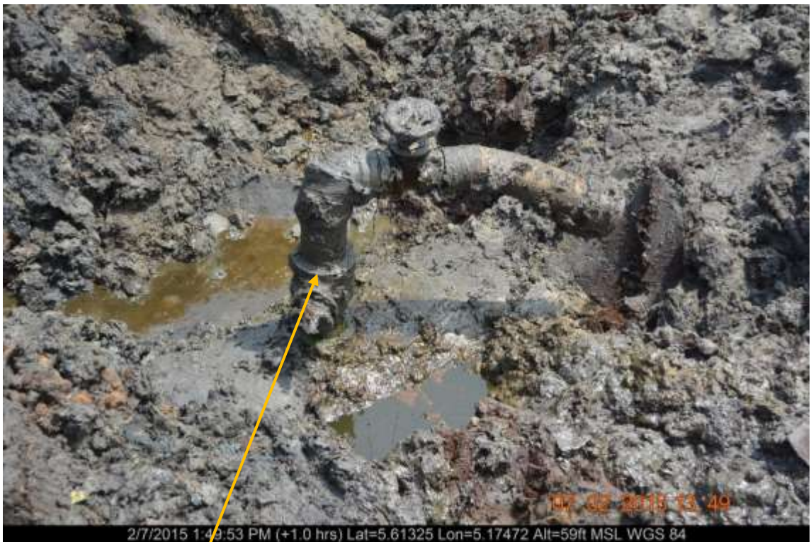
Close-up: Illegal fitting on 20" Otumara-Escravos Pipeline at Ugboegungun. Picture was taken during Joint Investigation of 7 th February 2015.
