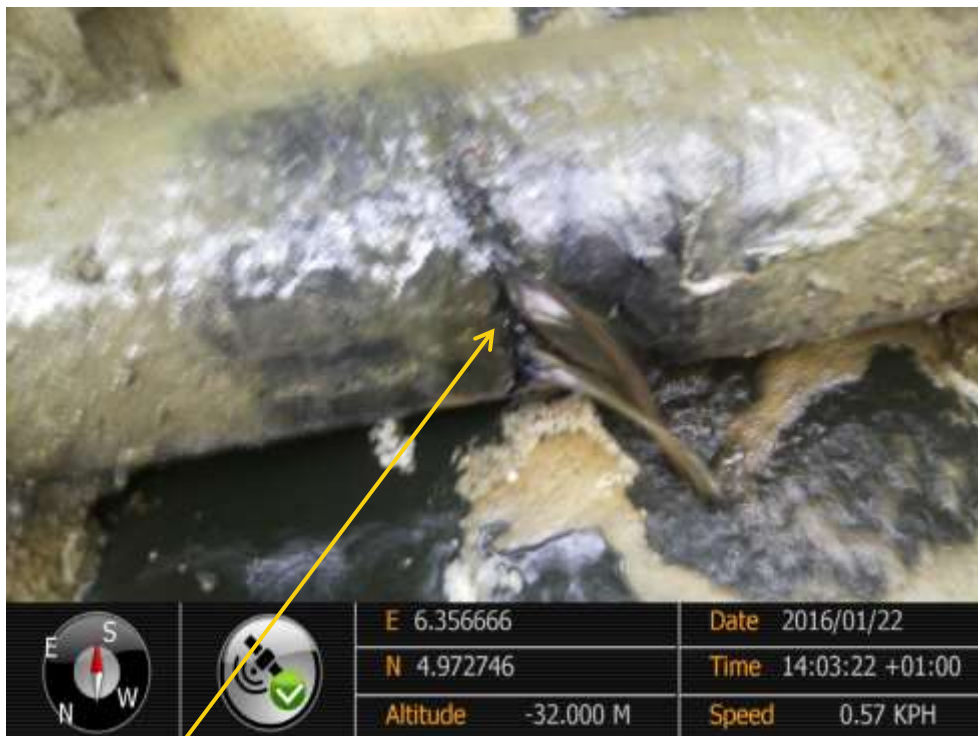
Close-up: Hacksaw cut on 8" Etelebou – KoloCreek Pipeline at Etegwe/Okutukutu. Picture was taken during Joint Investigation of 22 nd January 2016.
