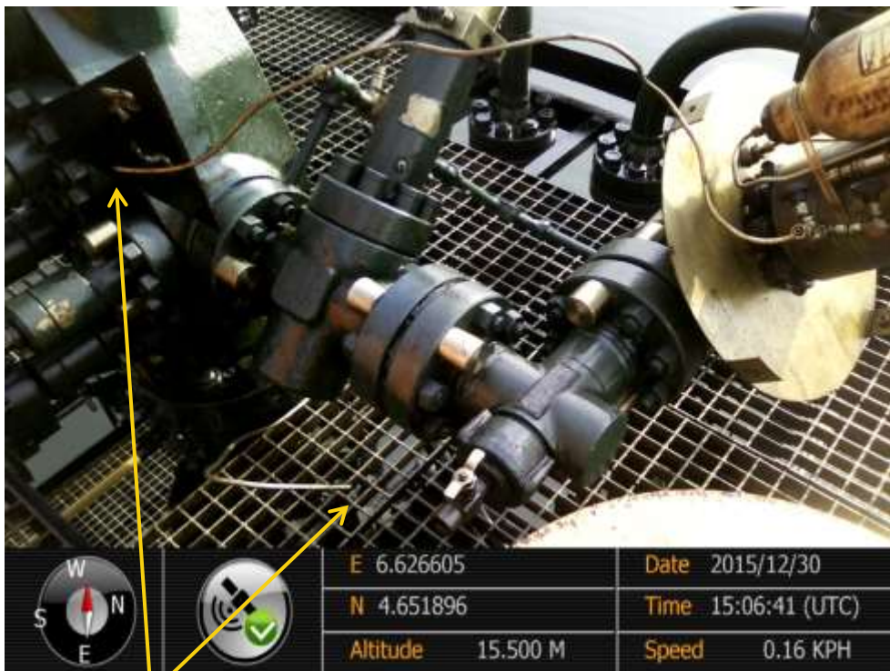
Close-up: Leak from cut ends of Sensing Line on Soku Well14S Wellhead at Soku. Picture was taken during Joint Investigation of 30 th December 2015.
