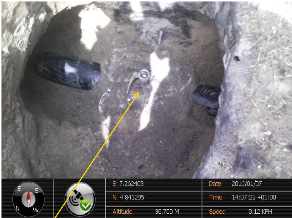
Close-up: Illegal fitting on Afam Well27 8" Flowline at Ayamandoki. Picture was taken during Joint Investigation of 7 th January 2016.
