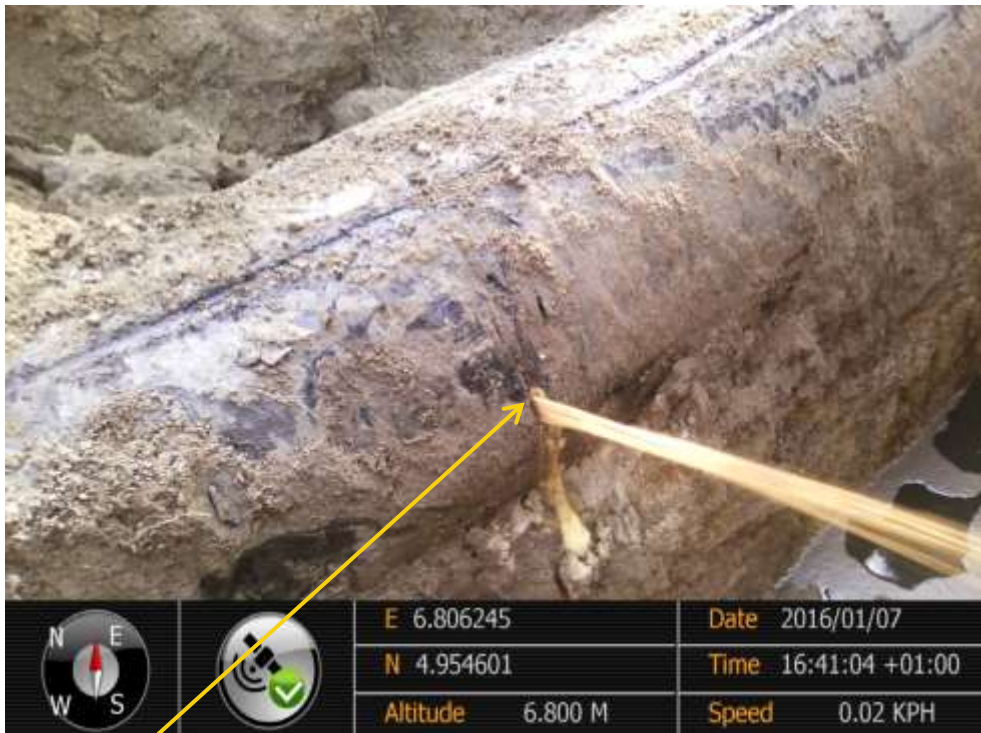
Close-up: Hacksaw cut on 20" Rumuekpe – Nkpoku Pipeline at Omukpobu-Ibaa. Picture was taken during Joint Investigation of 7 th January 2016.
