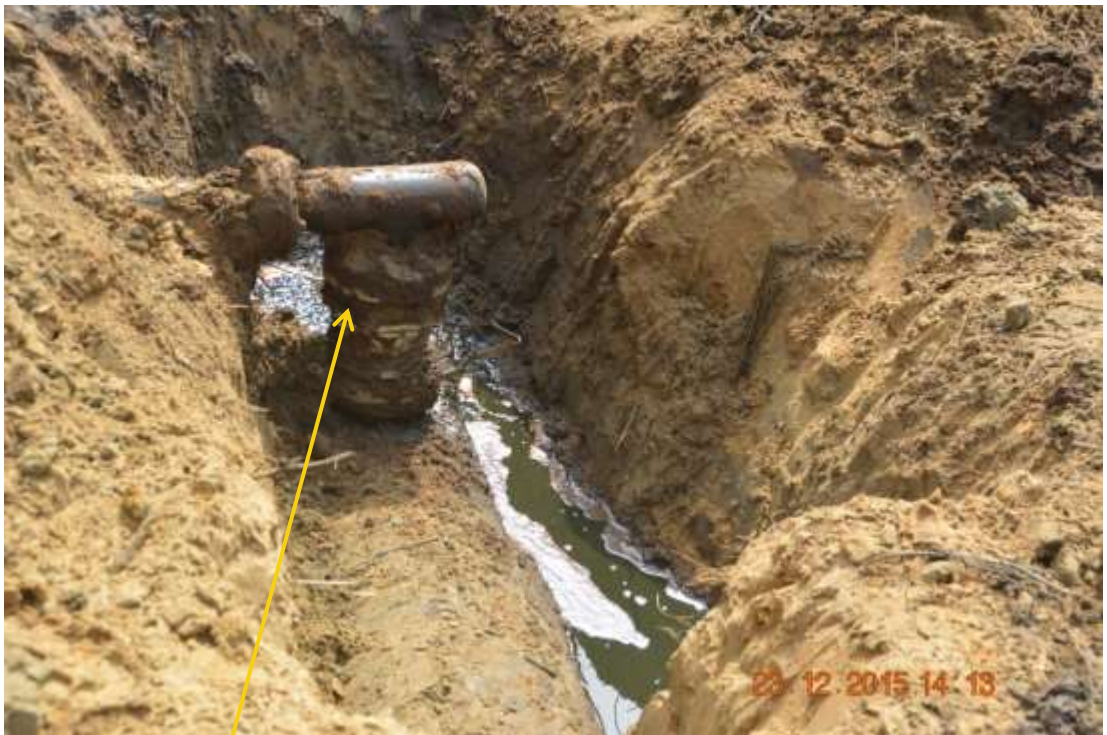
Close-up: Illegal fitting on 20" Otumara-Escravos Pipeline at Ogidigben. Picture was taken during Joint Investigation of 23 rd December 2015.
