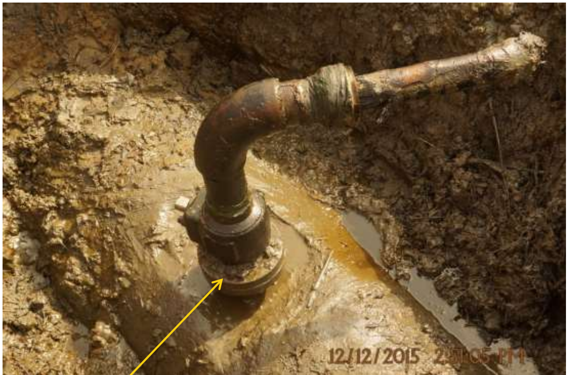
Close-up: Illegal fitting on 20" Otumara-Escravos Pipeline at Ugboegungun. Picture was taken during Joint Investigation of 12 th December 2015.
