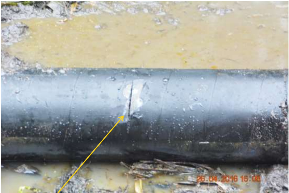
Close-up: Hacksaw cut on 6" Seibou Bulkline4 at Azagbene. Picture was taken during Joint Investigation of 26 th April 2016.
