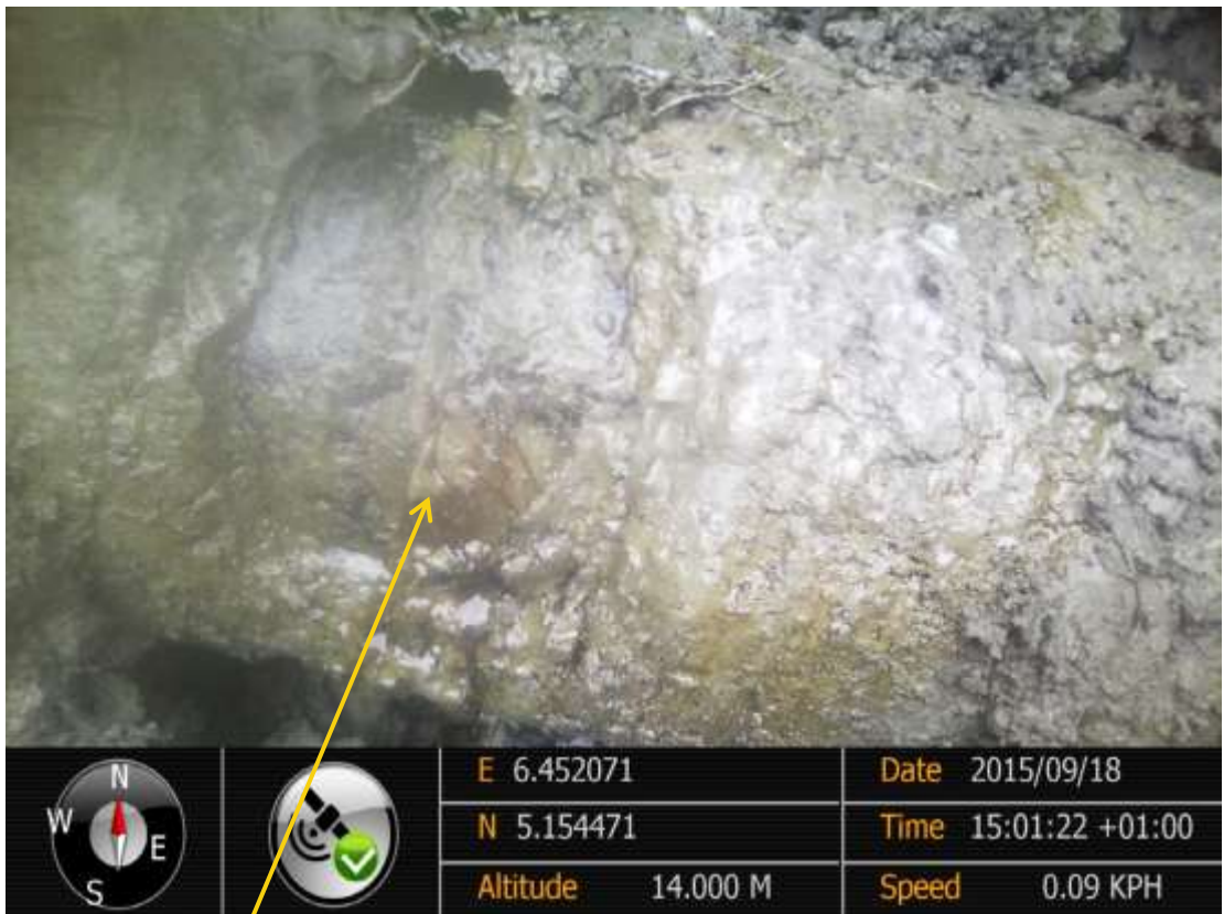
Close-up: Hacksaw cut on 12" Adibawa – Okordia Pipeline at Ikarama. Picture was taken during Joint Investigation of 18 th September 2015.
