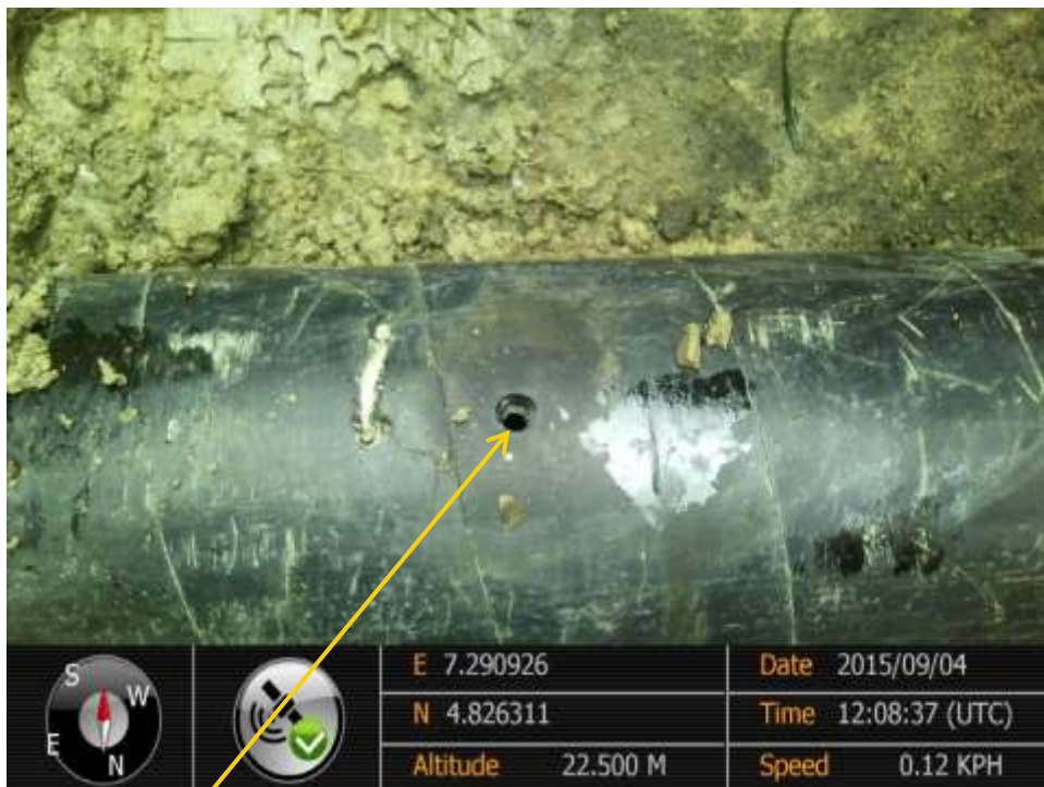
Close-up : Drilled hole on 8" Afam Well25 Flowline at Egberu. Picture was taken during Joint Investigation of 4 th September 2015.
