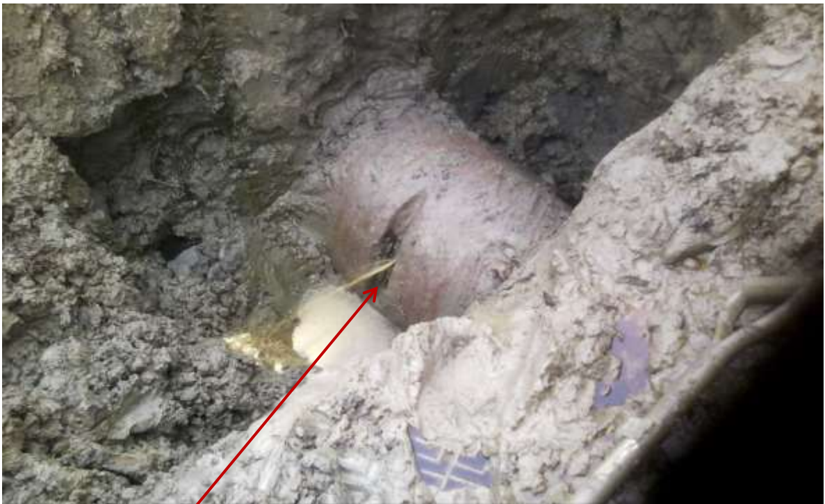
Close-up: Hacksaw cut on 20" Kolo Creek to Rumuekpe Pipeline at Odau. Picture was taken during Joint Investigation of 25 th August 2015.
