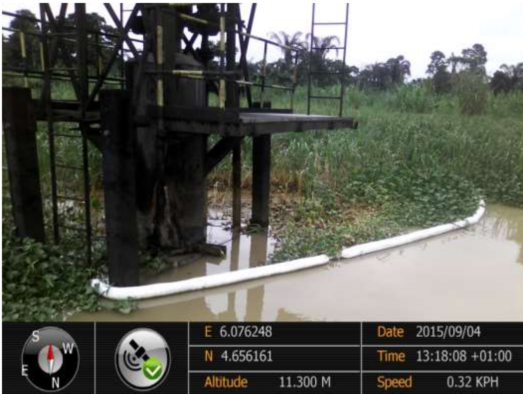
Overview: Part of spill impact on Diebu Creek Well1S Wellhead Right of Way at Peremabiri. Picture was taken during Joint Investigation of 4 th September 2015.
