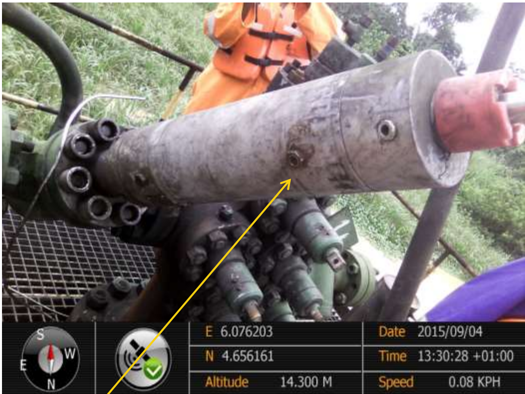
Close-up: Location of missing Cameron Control Unit on Diebu Creek Well1S Wellhead at Peremabiri. Picture was taken during Joint Investigation of 4 th September 2015.
