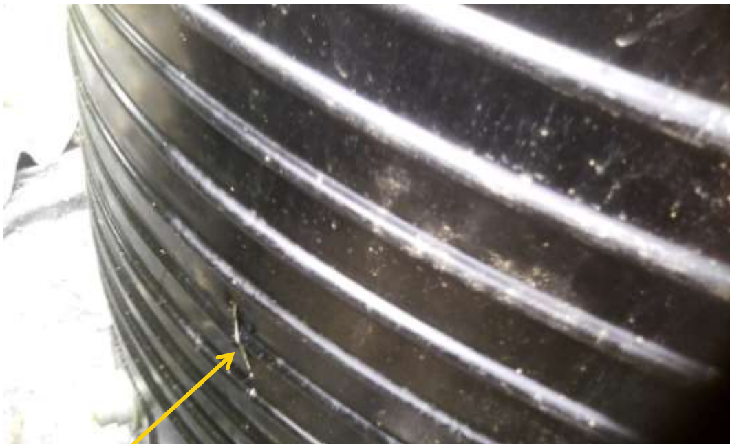
Close-up: Cut by unknown persons on Oil Storage Tank at Obedum Evacuation Plant. Picture was taken during Joint Investigation of 26 th August 2015.
