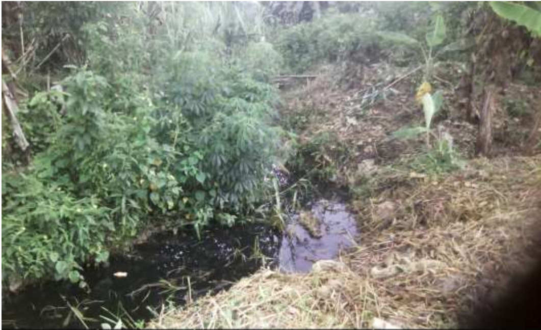
Overview: Part of spill impact around Obedum Evacuation Plant. Picture was taken during Joint Investigation of 26 th August 2015.
