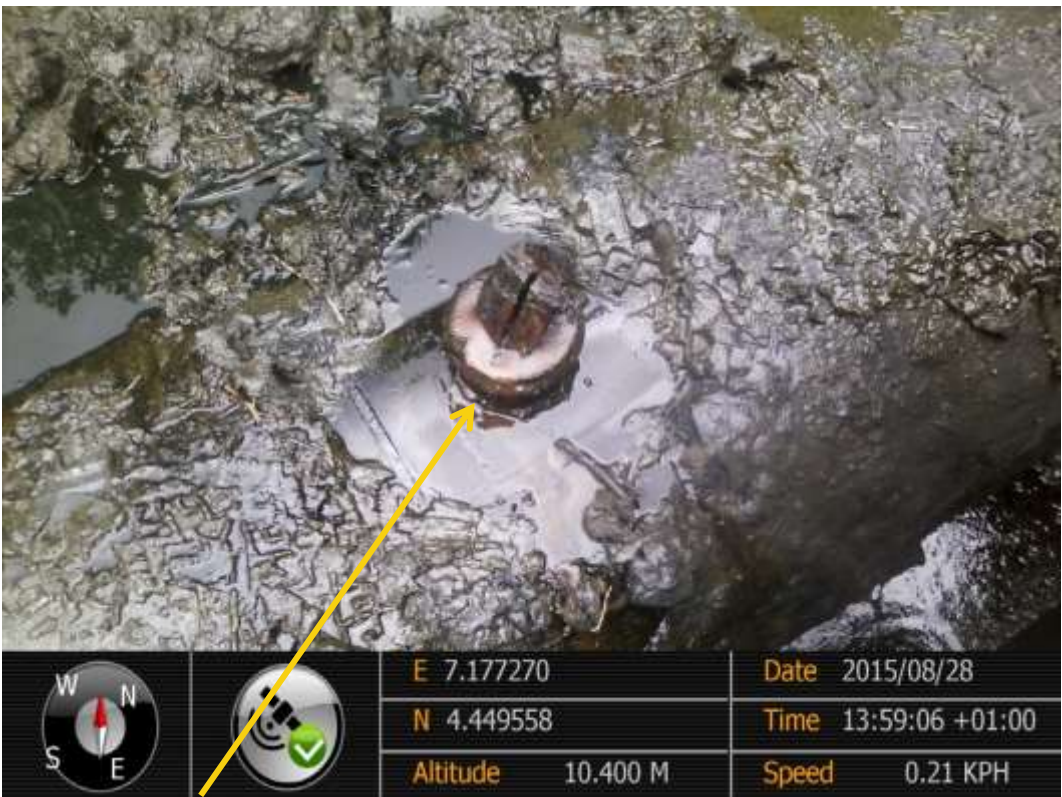
Close-up: Illegal fitting on 28" Bomu-Bonny Pipeline at Ayaminima. Picture was taken during Joint Investigation of 28 th August 2015.
