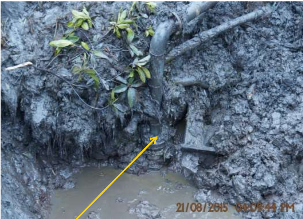
Close-up: Illegal fitting on 16" Tunu – Brass Creek Pipeline at Agbidiana. Picture was taken during Joint Investigation of 21 st August 2015.
