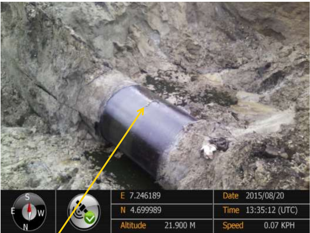
Close-up: Hacksaw cut on 28" Nkpoku - Bomu Pipeline at Gio. Picture was taken during Joint Investigation of 20 th August 2015.
