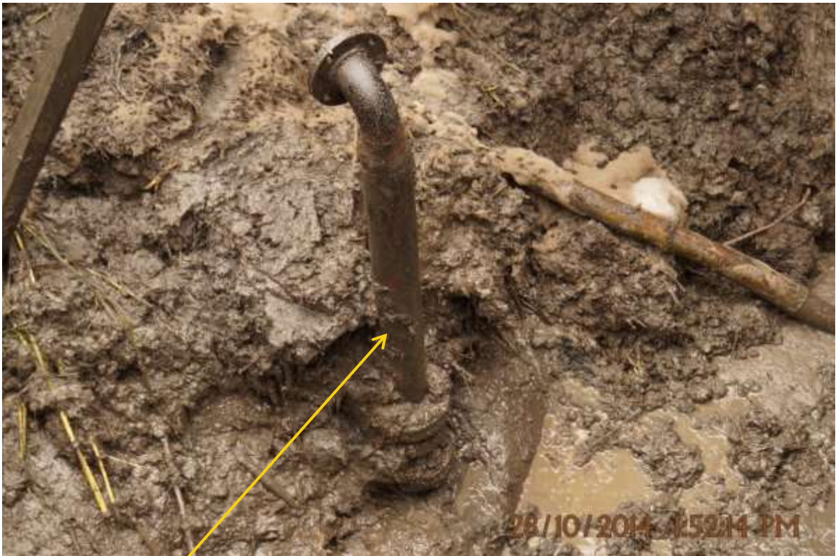
Close-up: Illegal fitting on 20" Opukushi – Brass Creek Pipeline at Peretourgbene. Picture was taken during Joint Investigation of 28 th October 2014.
