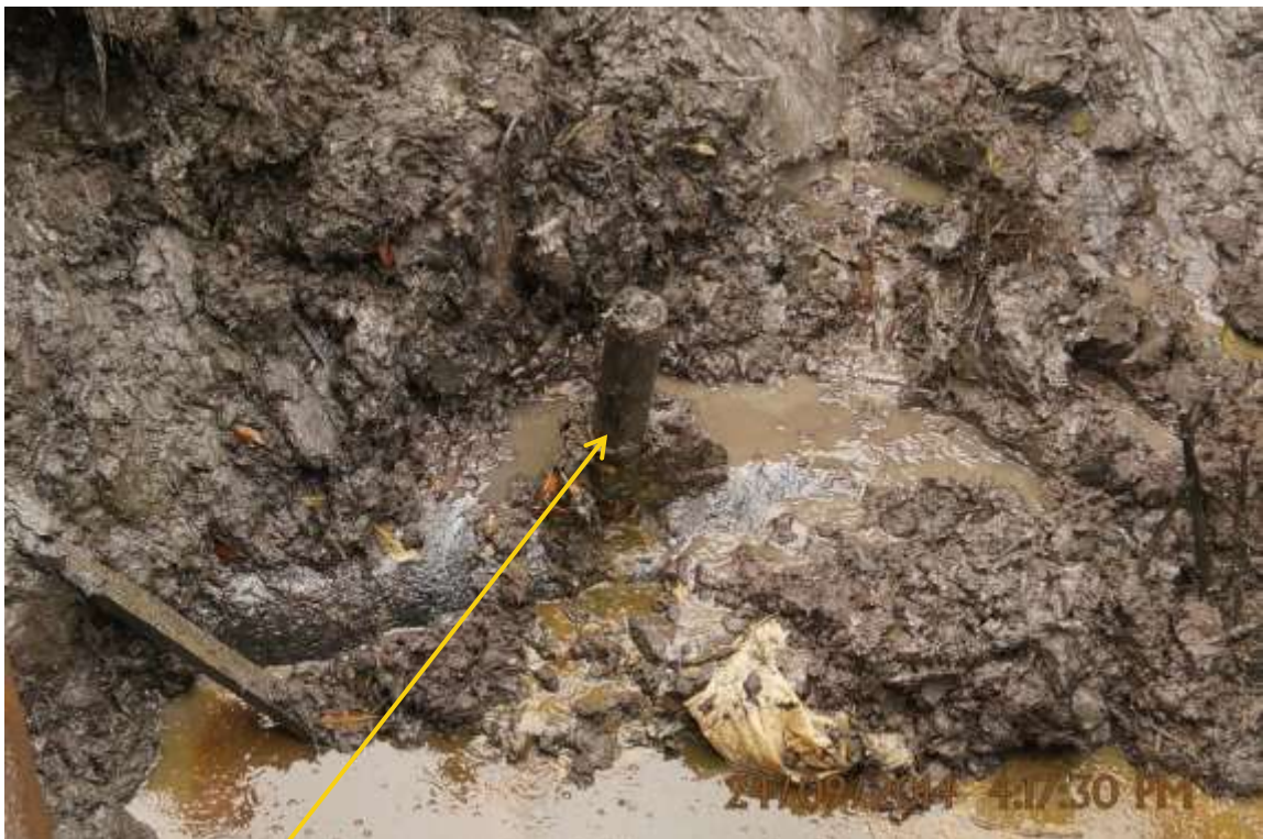
Close-up: Illegal fitting on 16" Tunu-Brass Creek Pipeline at Agbidiana. Picture was taken during Joint Investigation of 24 th September 2014.
