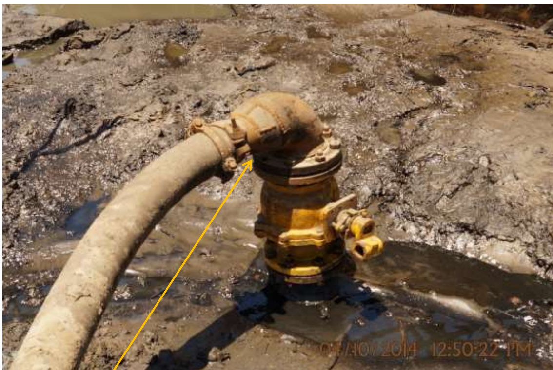
Close-up: Illegal fitting on 48" Forcados Crude Oil Export Pipeline at Ogulagha. Picture was taken during Joint Investigation of 4 th October 2014.
