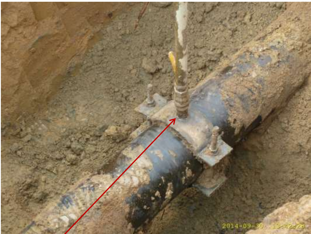
Close-up: Illegal fitting on 8" Umuechem-Nkpoku Pipeline at Omunwei. Picture was taken during Joint Investigation of 30 th September 2014.
