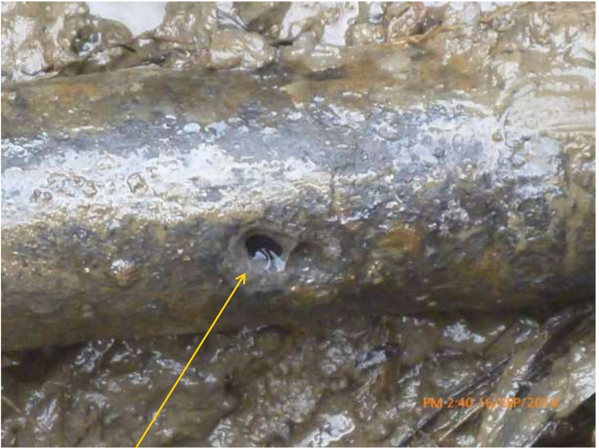
Close-up: Spill due to corrosion on Nun River Flowstation Sludge Discharge Line at Oporoma. Picture was taken during Joint Investigation of 16 th September 2014.
