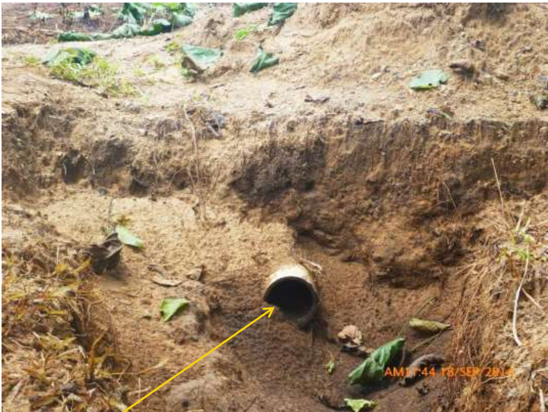
Close-up: Cut section of missing flowline on Ubie Well 4S Flowline at Idu-Ekpeye. Picture was taken during Joint Investigation of 18 th September 2014.
