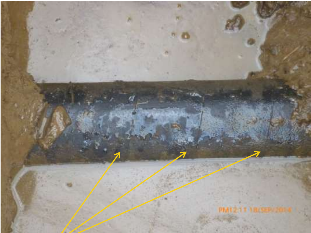
Close-up: Hacksaw cuts on Ubie Well 4S Flowline at Idu-Ekpeye. Picture was taken during Joint Investigation of 18 th September 2014.
