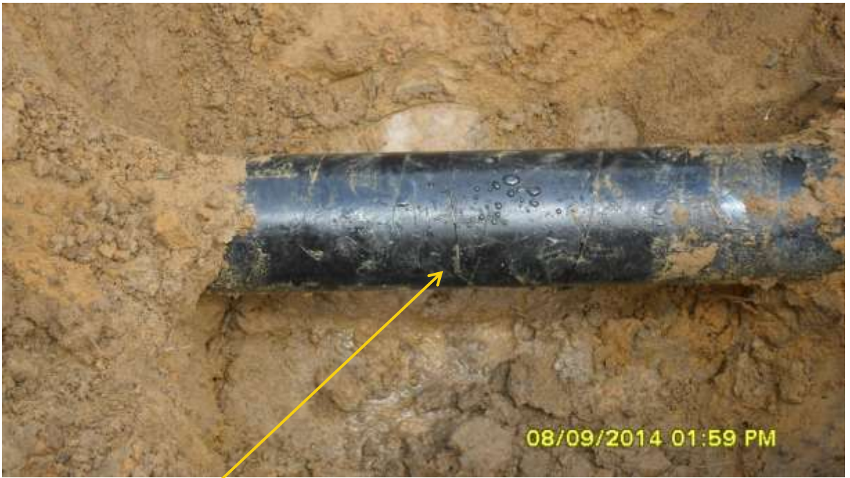
Close-up: Hacksaw cut on Ubie Well4S Flowline at Idu-Ekpeye. Picture was taken during Joint Investigation of 8 th September 2014.
