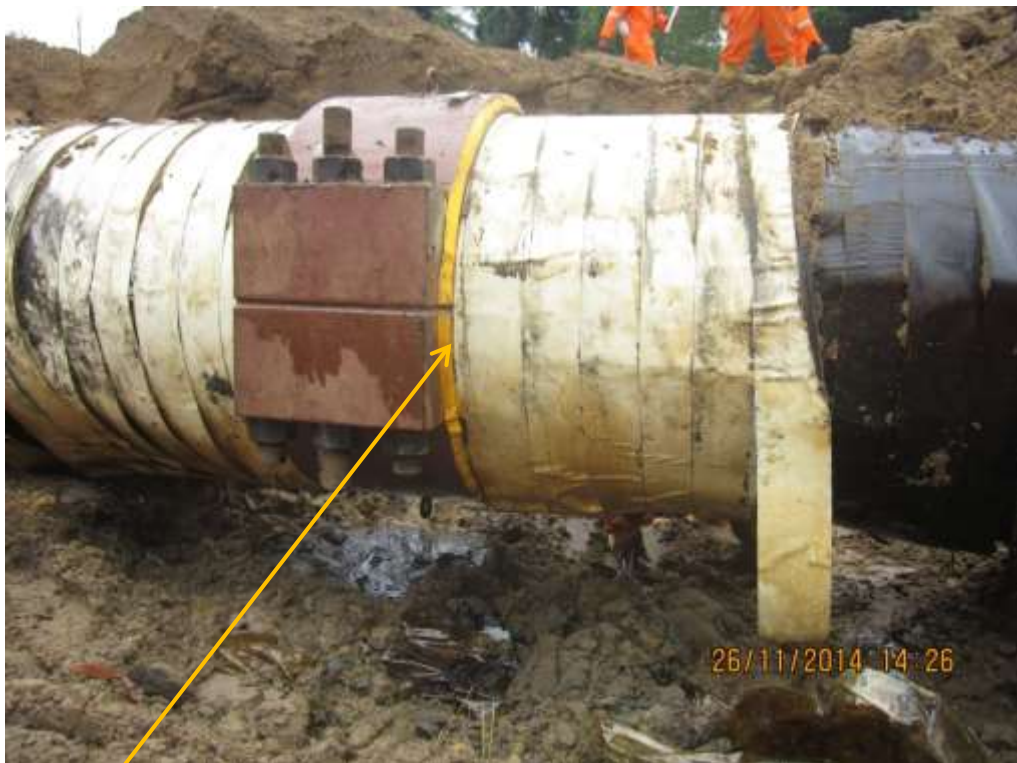
Close-up: Spill due to failed clamp on 28" Nkpoku-Bomu Pipeline at Ekporo. Picture was taken during Joint Investigation of 26 th November 2014.
