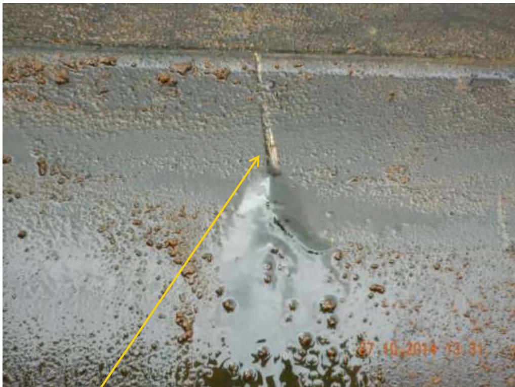
Close-up: Hacksaw cut on 18" Assa-Rumuekpe Pipeline at Egbeda. Picture was taken during Repair operations on 27 th November 2014.
