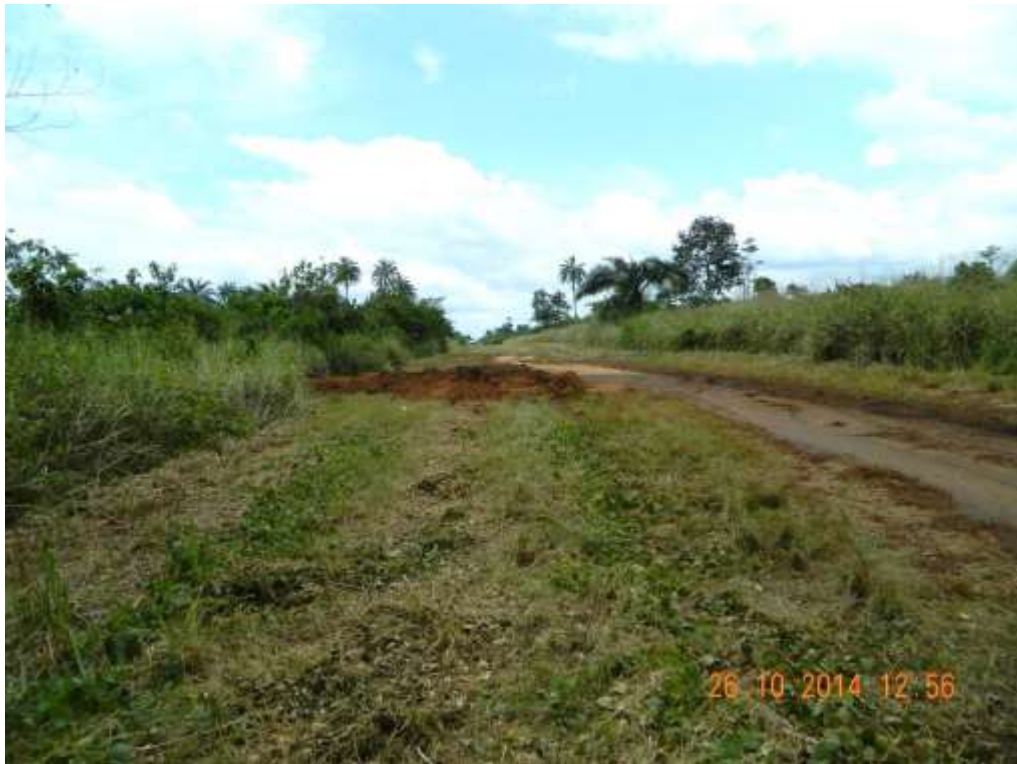
Overview: Part of spill impact on 18" Assa-Rumuekpe Pipeline at Egbeda. Picture was taken during Joint Investigation of 26 th November 2014.
