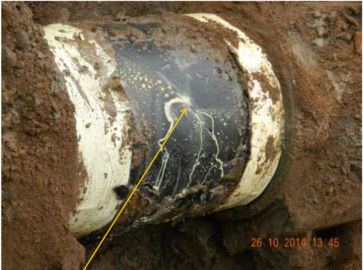
Close-up: Hacksaw cut on 18" Assa-Rumuekpe Pipeline at Egbeda. Picture was taken during Joint Investigation of 26 th November 2014.
