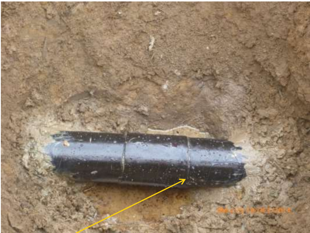
Close-up: Failed weld on 4" Agbada 2 Well2 Gaslift Flowline at Omuohia. Picture was taken during Joint Investigation of 19 th October 2014.
