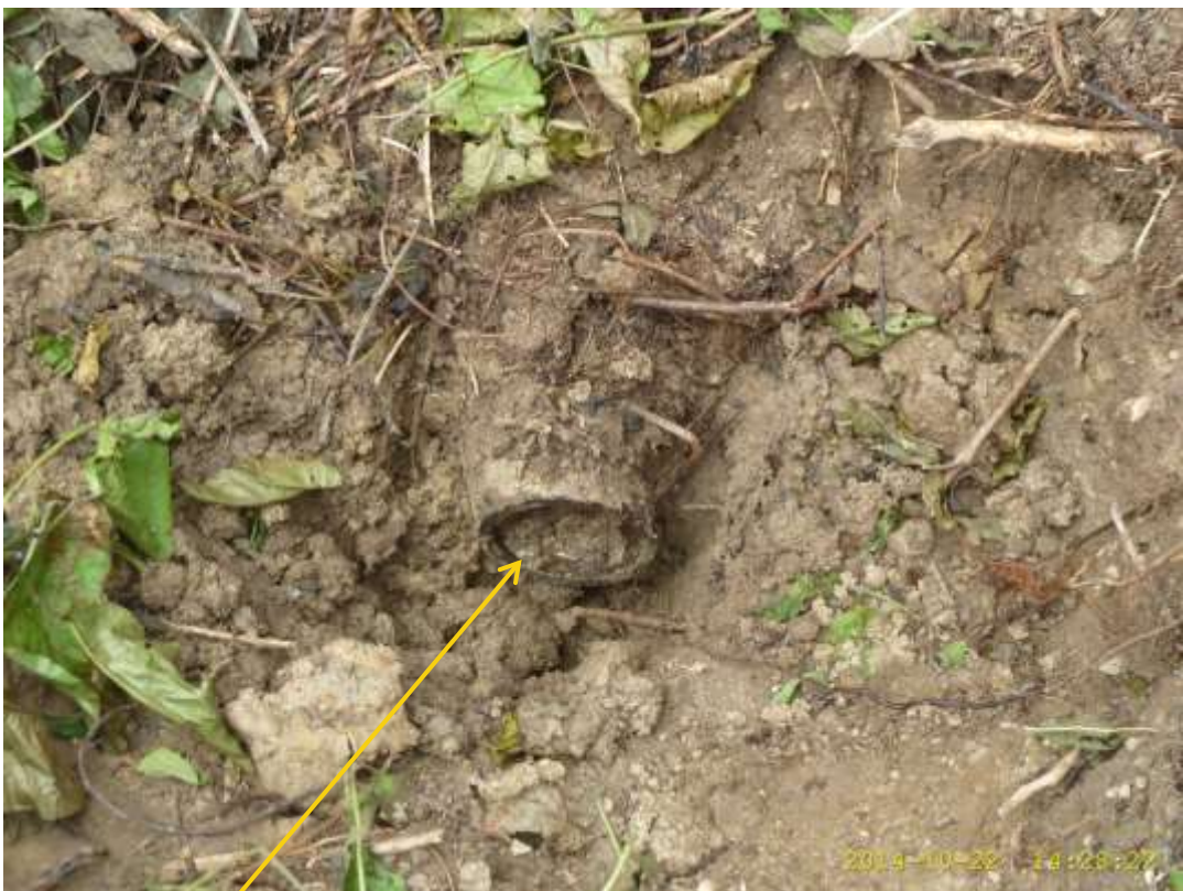
Close-up: Cut section of 4" KoloCreek Well3T Flowline at Otusega. Picture was taken during Joint Investigation of 22 nd October 2014.
