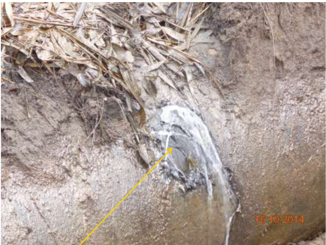
Close-up: Hacksaw Cut on 28" Nkpoku – Bomu Pipeline at Gio. Picture was taken during Joint Investigation of 16 th October 2014.
