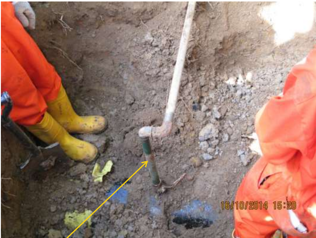
Close-up: Illegal fitting on 12" Imo River – Ogale Pipeline at Owaza. Picture was taken during Joint Investigation of 16 th October 2014.
