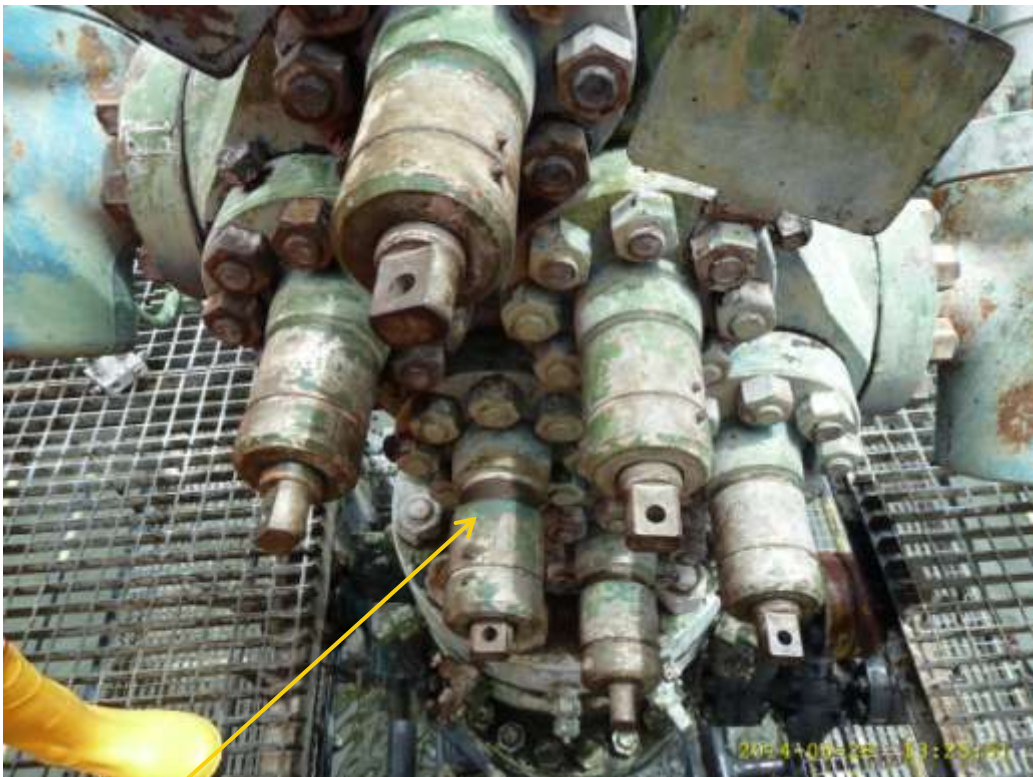
Close-up: Tampered valve on Soku Well21SL Wellhead slot at Russia. Picture was taken during Joint Investigation of 28 th May 2014.
