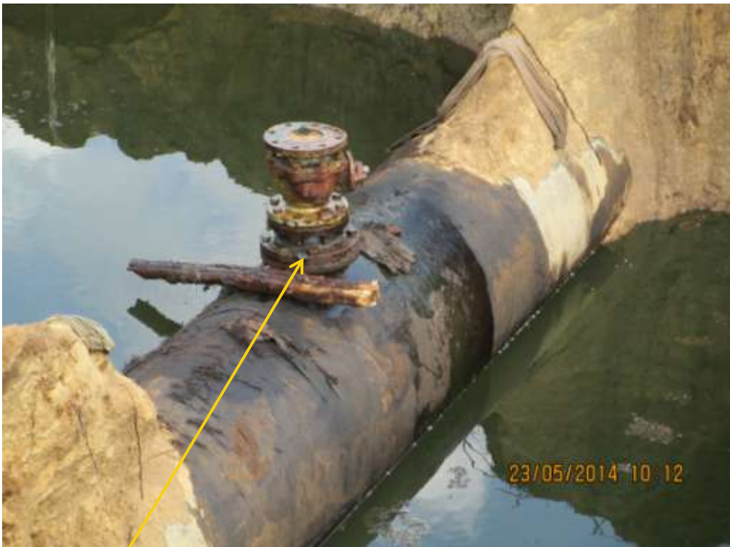
Close-up: Illegal fitting on 28" Nkpoku-Bomu Pipeline at Ekporo. Picture was taken during Joint Investigation of 23 rd May 2014.
