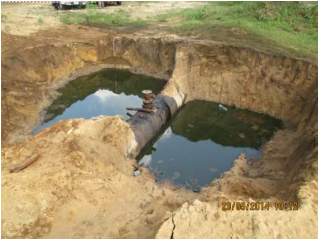
Overview: Part of spill impact on 28" Nkpoku-Bomu Pipeline Right of Way at Ekporo. Picture was taken during Joint Investigation of 23 rd May 2014.
