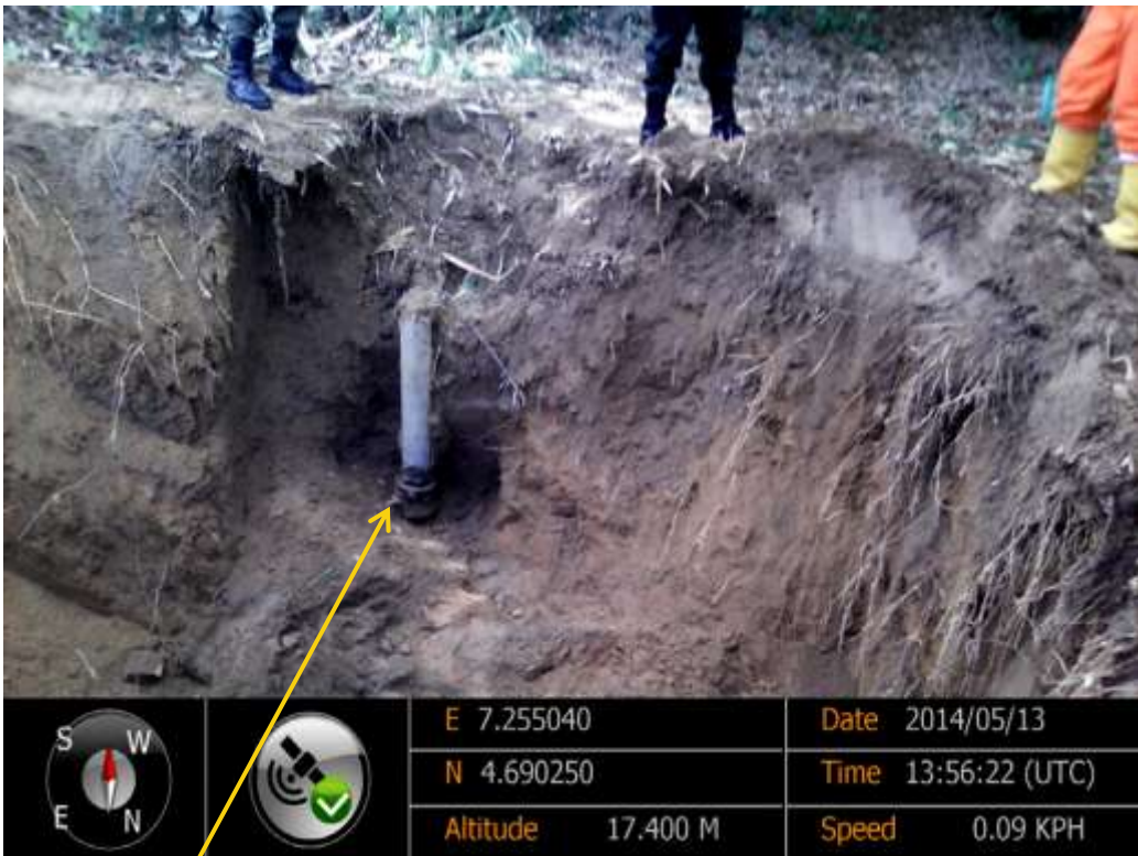
Close-up: Illegal fitting on 28" Nkpoku-Bomu Pipeline at B-Dere. Picture was taken during Joint Investigation of 13 th May 2014.
