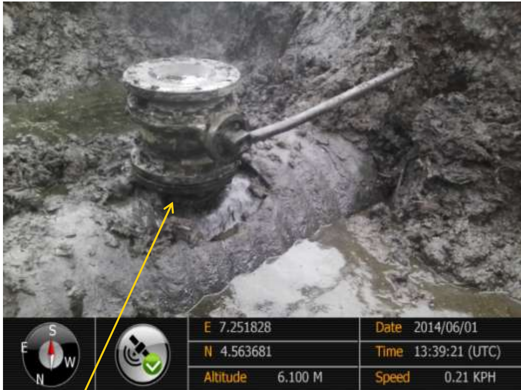
Close-up: Illegal fitting on 28" Bomu-Bonny Pipeline at Bodo City. Picture was taken during Joint Investigation of 1 st June 2014.
