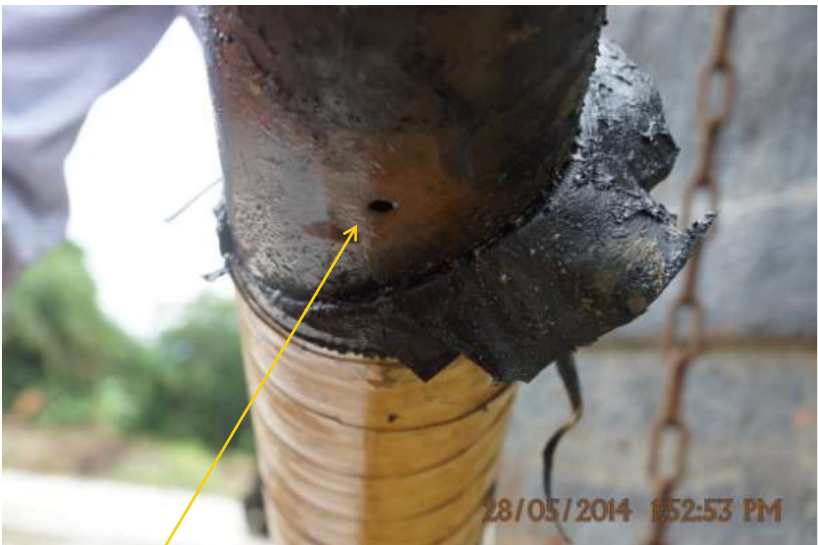
Close-up: Spill due to corrosion on Benisede –Akono Well1S Flowline at Ojobo. Picture was taken during Joint Investigation of 28 th May 2014.
