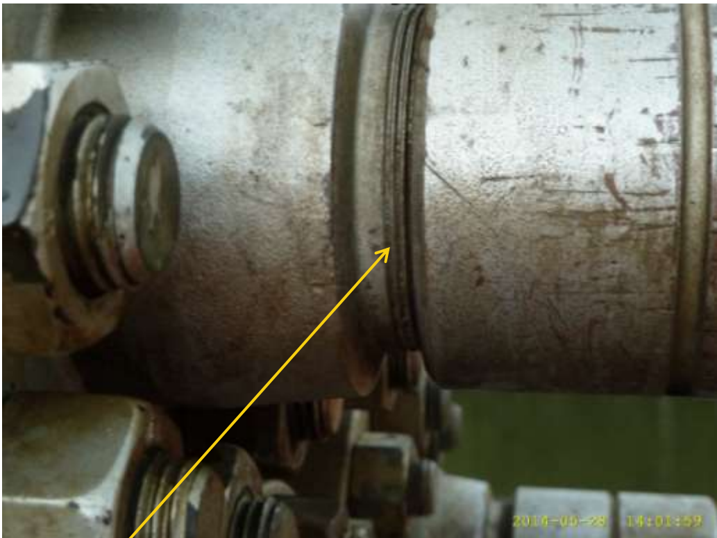
Close-up: Tampered valve on on Soku Well48L Wellhead slot at Russia. Picture was taken during Joint Investigation of 28 th May 2014.
