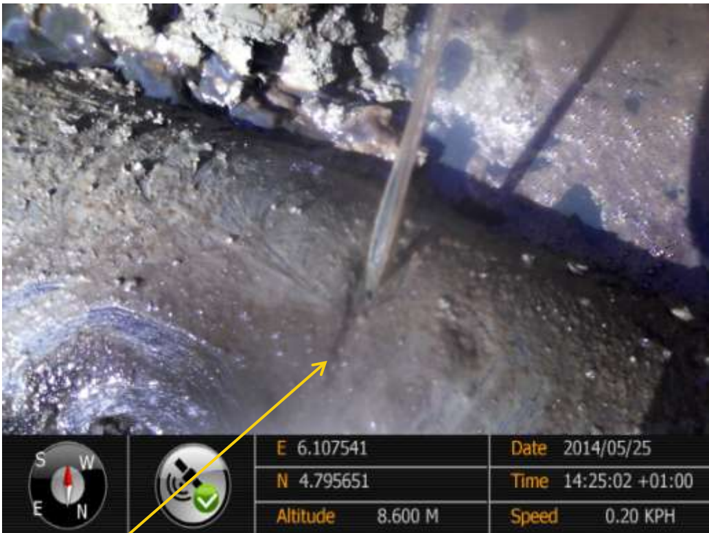
Close-up: Hacksaw cut on 10" Diebu Creek – NunRiver Pipeline at Oporoma. Picture was taken during Joint Investigation of 25 th May 2014.
