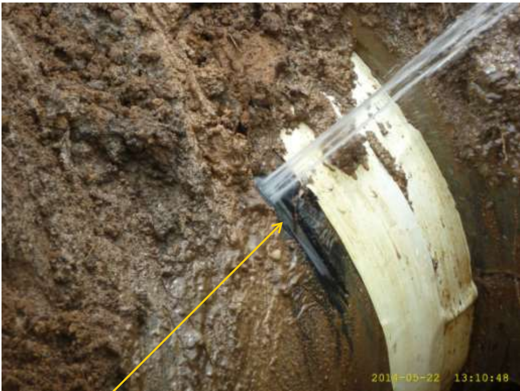
Close-up: Hacksaw cut on 28" Nkpoku-Bomu Pipeline at Biara. Picture was taken during Joint Investigation of 22 nd May 2014.
