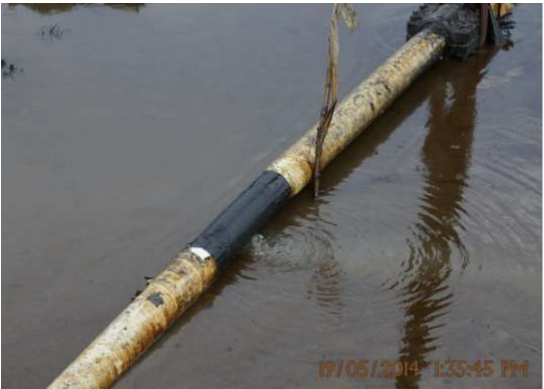
Close-up: Bubbling from pinhole on Otumara Well22L Flowline at Ugboegungun. Picture was taken during Joint Investigation of 19 th May 2014.
