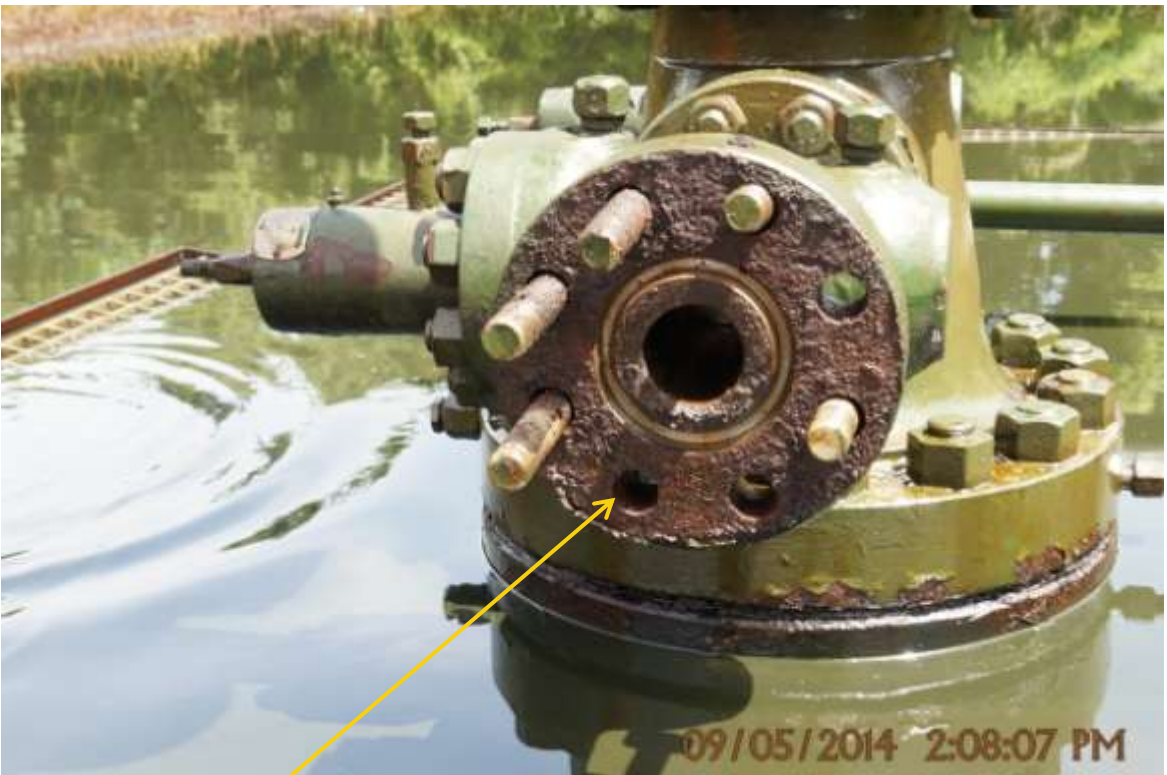
Close-up: Tampered valve on Yokri Wellhead79 at Sokebolou. Picture was taken during Joint Investigation of 9 th May 2014.
