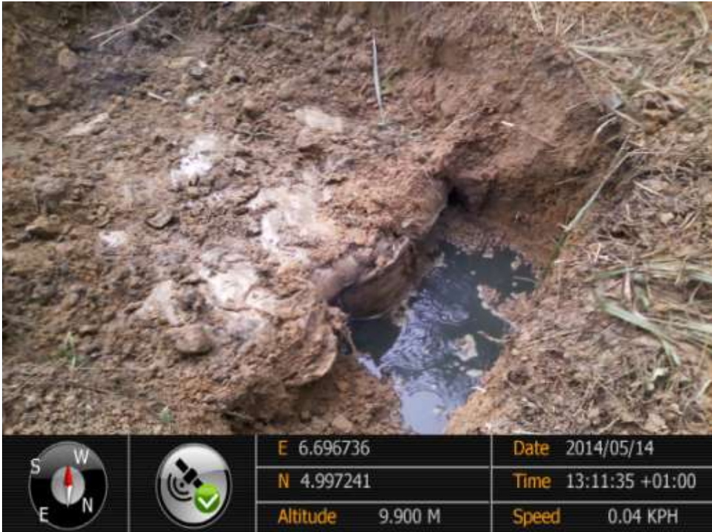
Overview: Spill impact on 8" Mininta-Rumuekpe Pipeline Right of Way at Rumuekpe. Picture was taken during Joint Investigation of 14 th May 2014.
