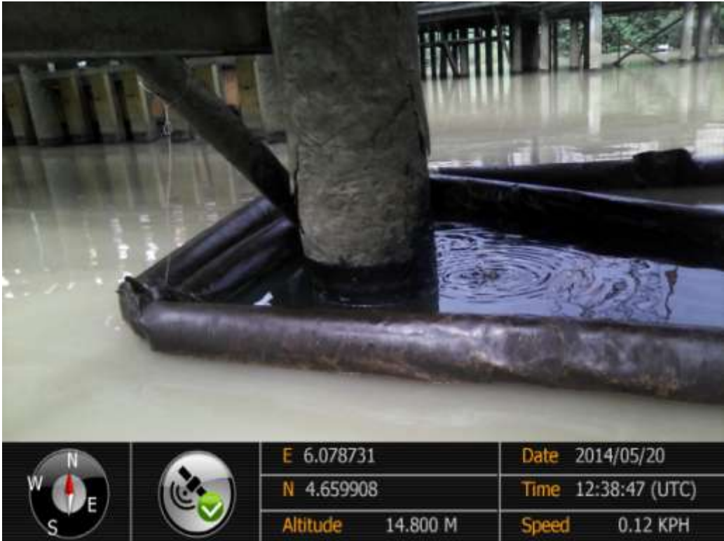
Overview: Spill impact on Diebu creek Flowstation Right of Way at Peremabiri. Picture was taken during Joint Investigation of 20 th May 2014.
