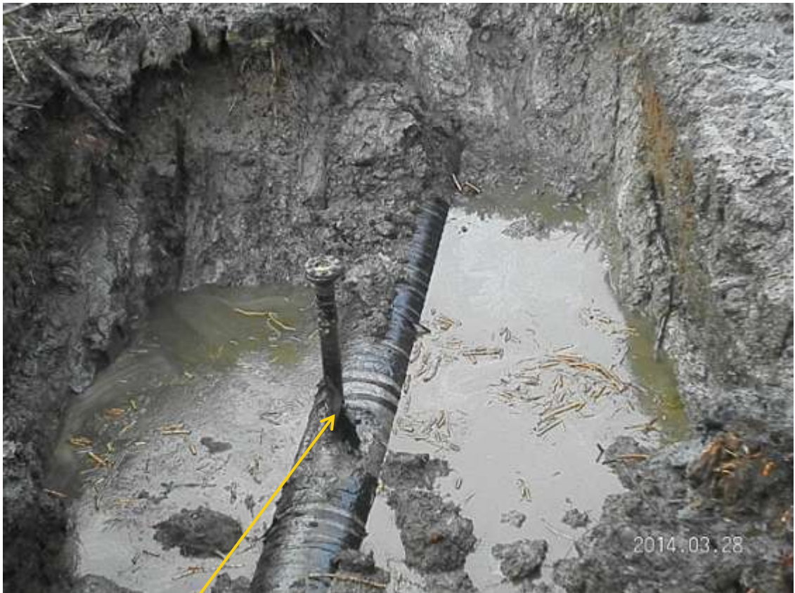
Close-up: Illegal fitting on old 24" Nembe Creek Pipeline at Twoni. Picture was taken during Joint Investigation of 28 th March 2014.
