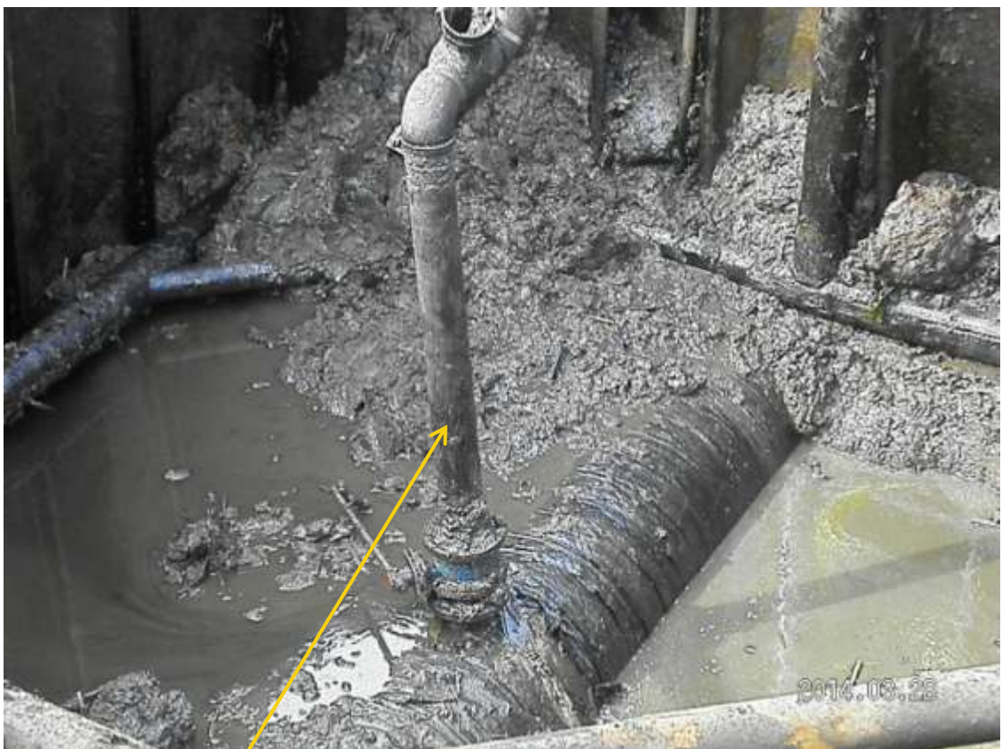
Close-up: Illegal fitting (non-leaking) on old 24" Nembe Creek Pipeline at Twoni. Picture was taken during Joint Investigation of 28 th March 2014.
