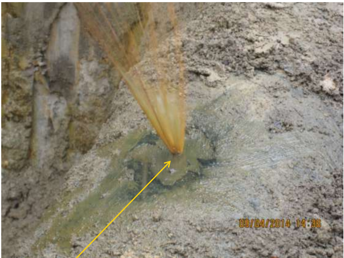
Close-up: Drilled hole on 20" Rumuekpe – Nkpoku Pipeline at Omusunu/Ibaa. Picture was taken during Joint Investigation of 9 th April 2014.
