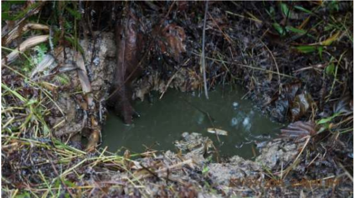
Overview: Part of spill impact on 12" Benisede – Brass Creek Pipeline right of way at Ojobo. Picture was taken during Joint Investigation of 27 th March 2014.
