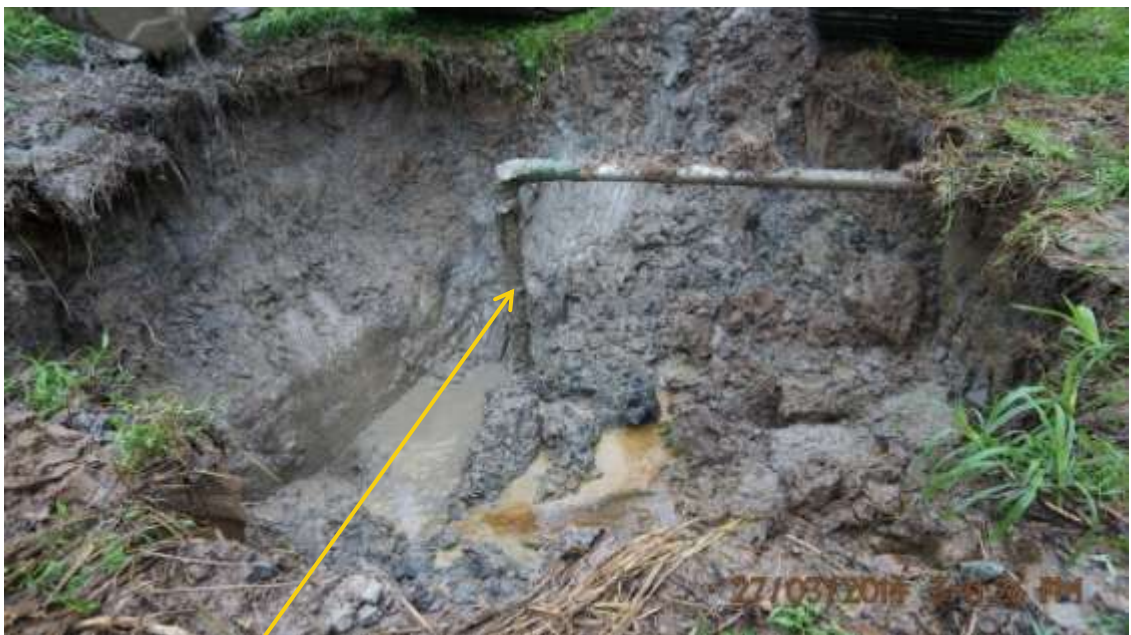
Close-up: Illegal fitting on 12" Benisede – Brass Creek Pipeline at Ojobo. Picture was taken during Joint Investigation of 27 th March 2014.
