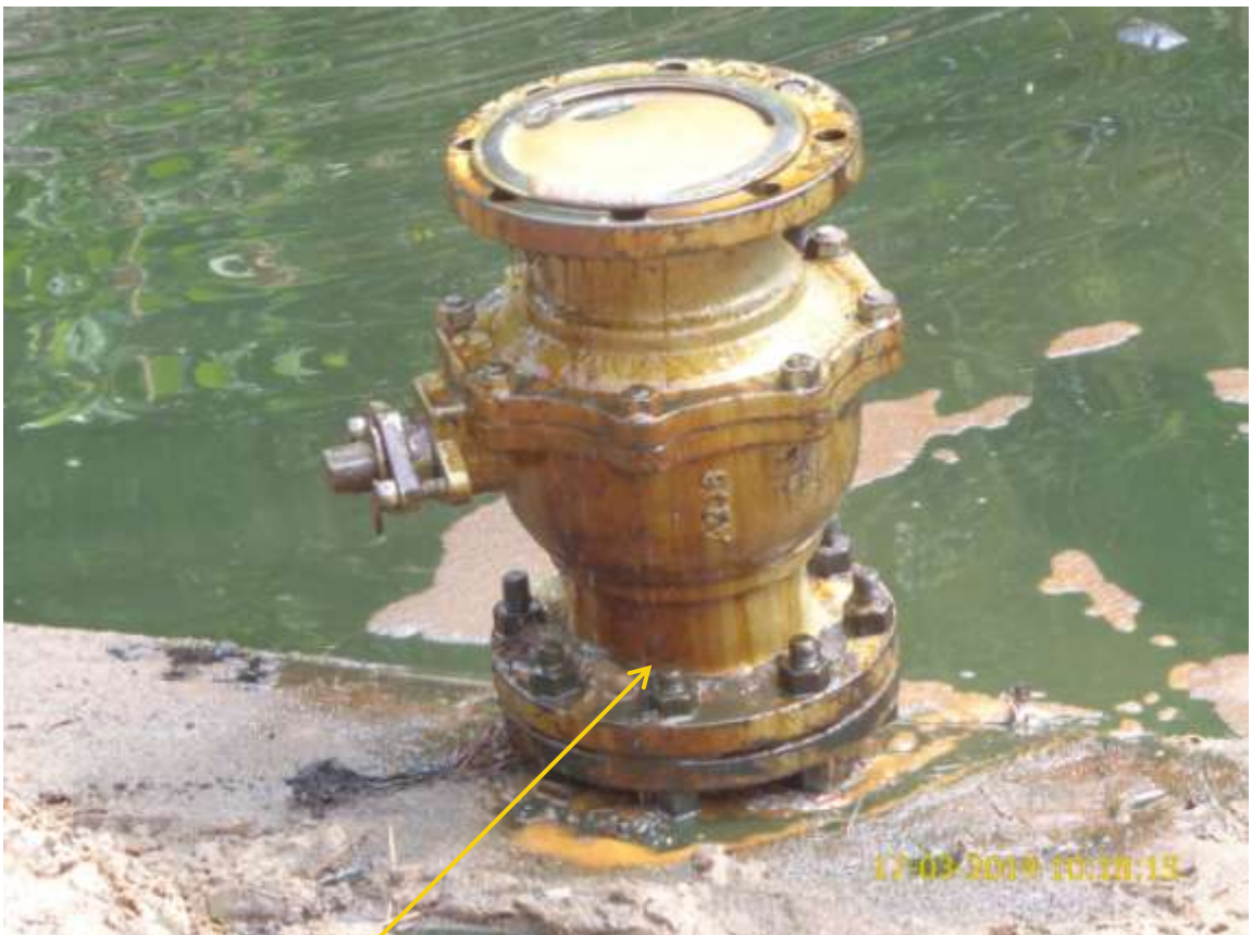
Close-up: Illegal fitting on 28" Nkpoku-Bomu Pipeline at B-Dere. Picture was taken during Joint Investigation of 17 th March 2014.
